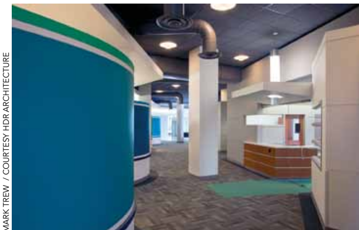
Showing the aesthetics of open plenum with exposed pipes, ducts, and vents is HDR Architecture's ceiling design for a University of Texas M.D. Anderson Cancer Center research building in Houston.
